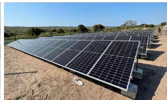
South Africa System Capacity: 580kW
