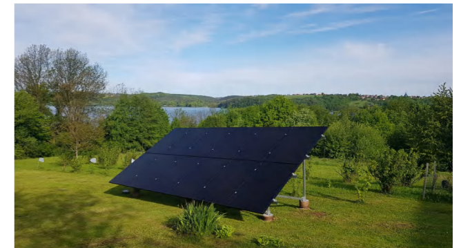
Poland System Capacity: 10kW
