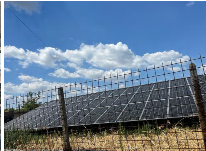
Poland System Capacity: 350kW
